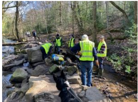
Great teamwork. Cement mixers, cement transporters and wall builders all work together to achieve the goal. Photo: Roger Kite
