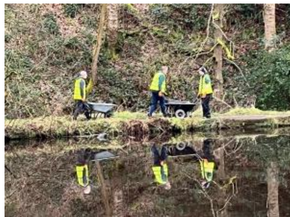
How to double the workforce: Footpath material is carefully barrowed around Hind Wheel in this reflective photo
