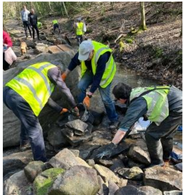
First goit section being repaired. In the background, a family with a dog attempting to negotiate the damaged footpath despite RVCG path closure signs!
