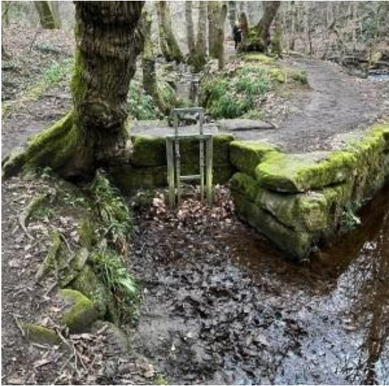
The Wolf Goit completely blocked with mud, shale, twigs and leaves following a winter storm.
