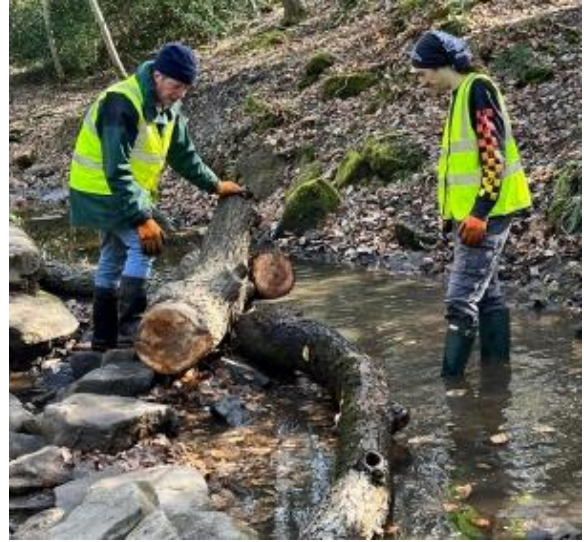
To begin with, a large tree had fallen across the goit and had to be sawn up and removed before repairs could begin.
