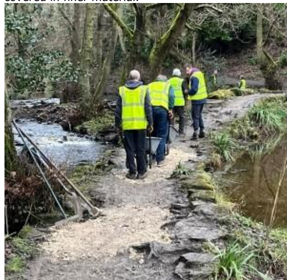
The footpath voids at Hind now repaired to make a more comfortable and safe passage for its visitors.
