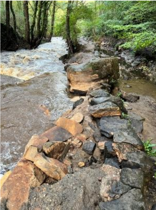
Oct 2023: Hind Wheel to Upper Cut footpath and goit wall severely damaged by the swollen river on the left leaving the goit on the right without water.
