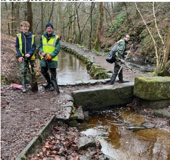
Frank Goit dug out by its proud volunteers and the water now free flowing into its dam. Photo: Graham Axelby
