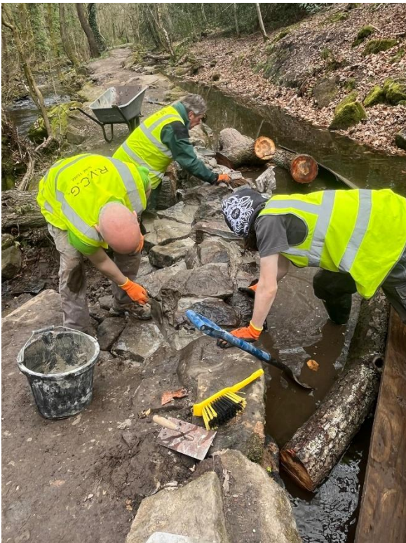
Day 2 volunteers, Father & son, Kevin and Ed McManus (front) and Gary Cliff (rear): The second larger section of goit wall in progress.
