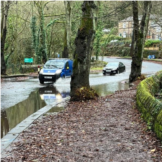
Glen Bridge at the S bend flooded following heavy rain despite the recent installation of twin gulleys.
