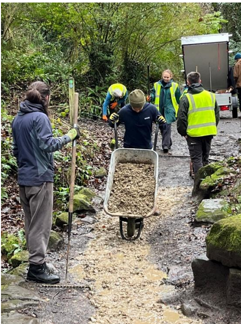
The sandstone is barrowed into place, raked smooth and then compacted with the RVCG vibrator.
