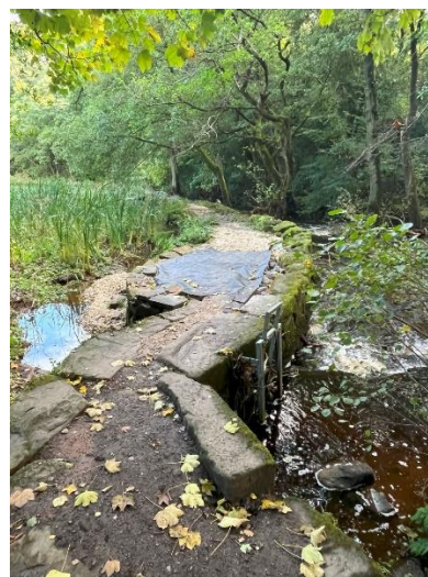
Sep 30 th The footpath topping washed straight into the dam. Fortunately, the dam wall remains intact.
