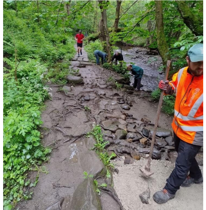
Sheffield City Council Ranger Ryan Atkin leading the footpath repairs at the end of May task day
