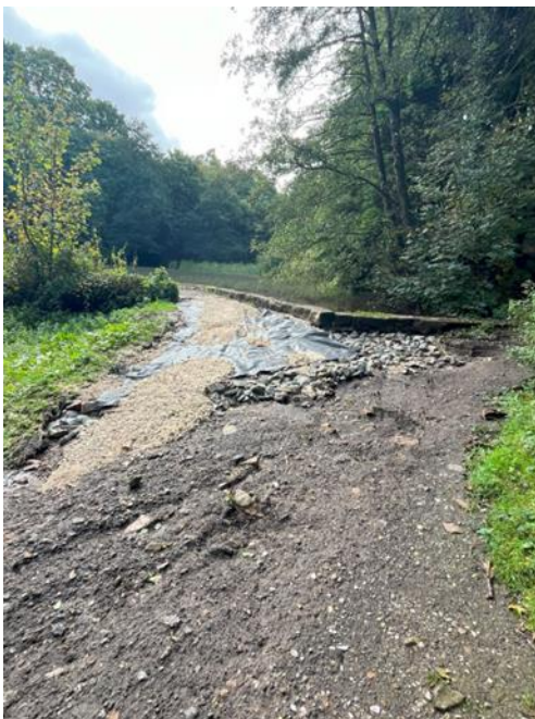
Sep 30 th washed away again in the recent flash flood
