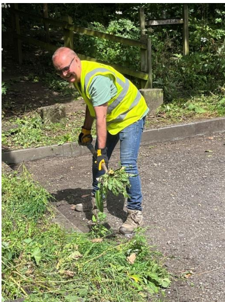
Clearing the undergrowth and verges (with a smile) at Rails Road car park (Rivelin Corn Mill)
