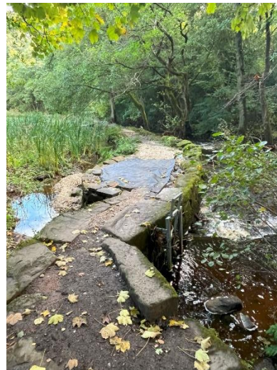
Sep 30 th The footpath topping washed straight into the dam. Fortunately, the dam wall remains intact.
