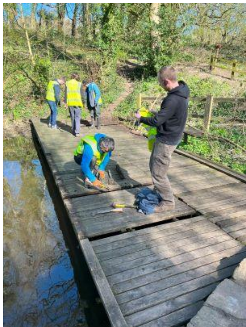
Task team volunteers replacing rotting timbers at Rivelin Corn Mill dipping platform
