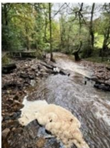
Swallow Goit Blockage and Weir Damage
