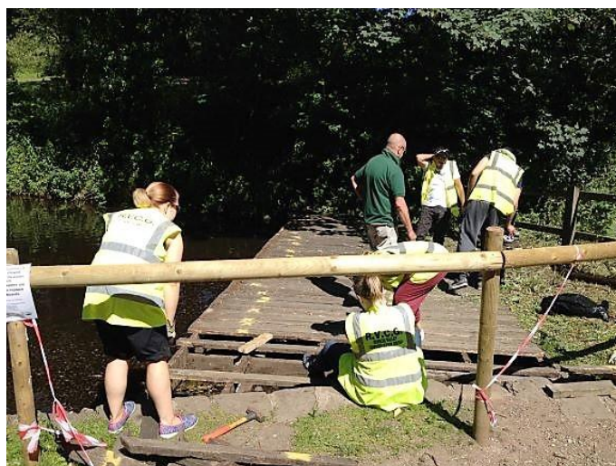
Figure 3 Volunteers from Virgin Media remove rotting boards from Rivelin Mill dipping platform in preparation for the RVCG Task Team to replace the boards on the following task day on the last Sunday in May
