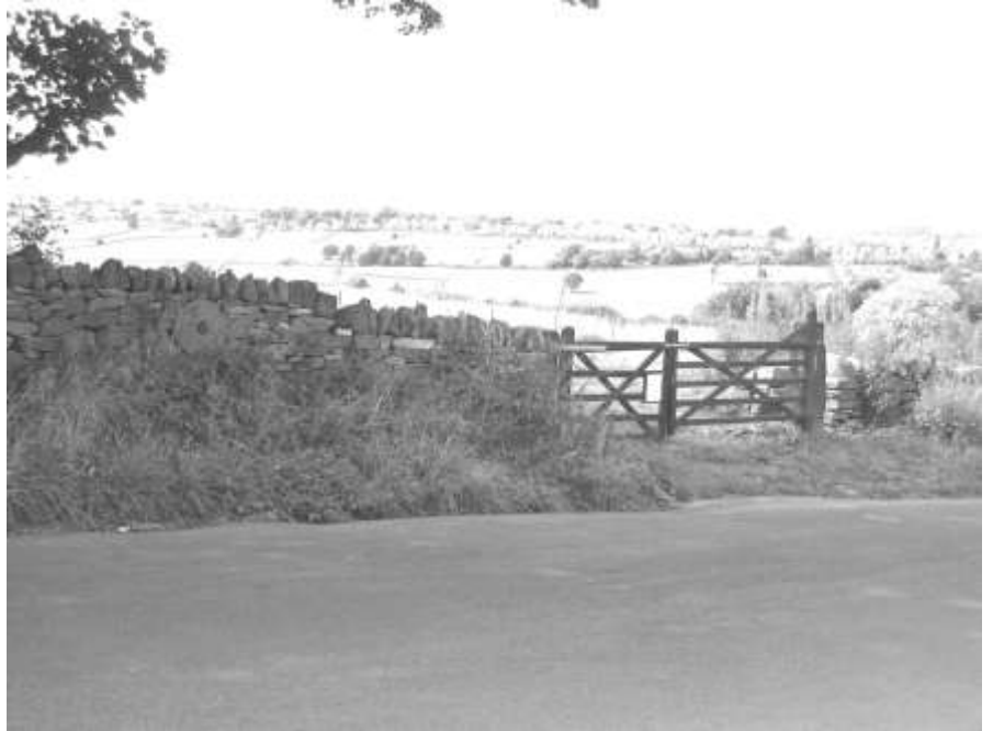
The newly reconstructed wall and top gate at Carver Fields off Hagg Lane
